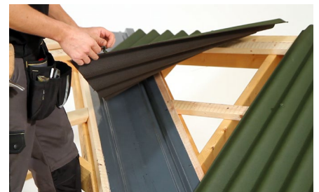
Positioning sheet The sheets are then positioned back on the roof, aligned square to the line of the roof sheets providing the minimum of 4cm drip edge into gutter.
