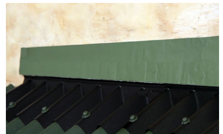
Apron cover flashing To allow for differential movement between the wall and the roof sections always use a separate wall cover flashing dressed into a prepared joint.
