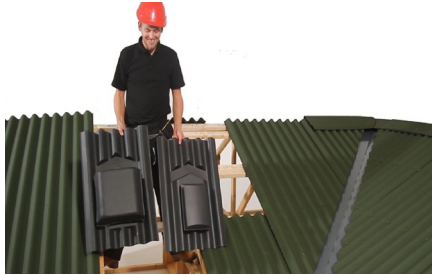
Basic verge detail Roof ventilators are available in two sizes to provide increased ventilation and should be used mid span on roof slope / lengths greater than 11m.
