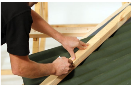
Marking sheet to valley Position the Onduline sheets up the line of the valley and mark out the cut line, allowing for a minimum of 4cm sheet drip edge into the valley gutter.
