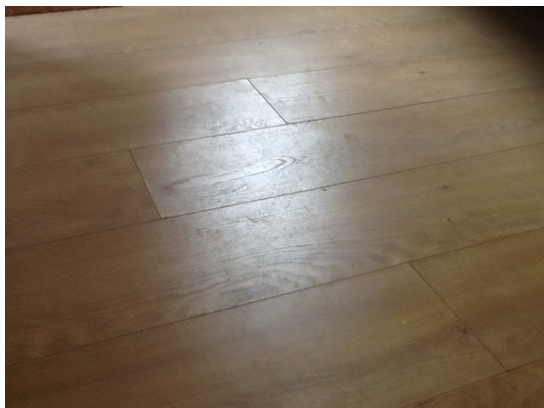
Incorrect cleaning agent/smears on the surface
