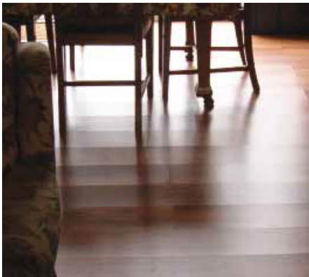
Inappropriate ventilation. Expansion gaps incorrect or lack of DPM (concrete subfloor)
