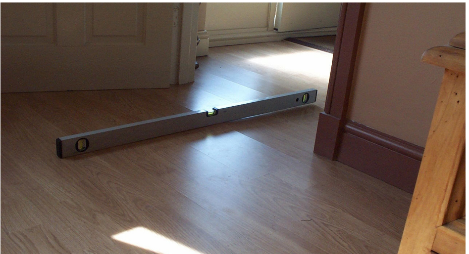
Non-observance of wall/boarder. No threshold joints between rooms
