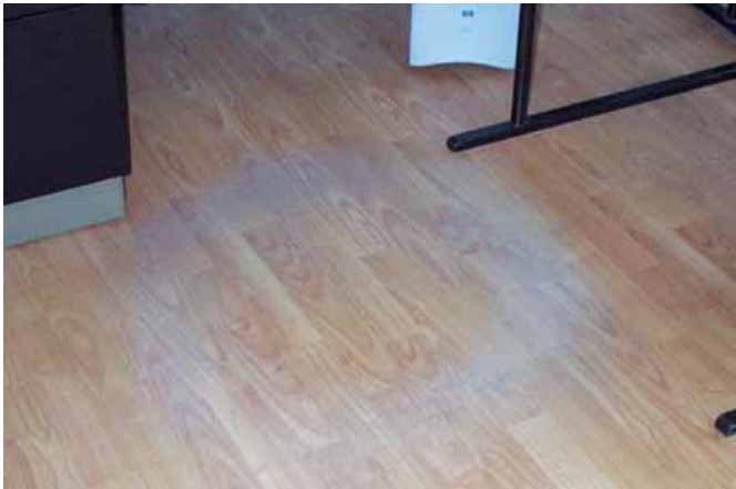
Abrasion caused by incorrect chair casters
