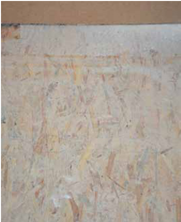
Unsuitable insulation material
