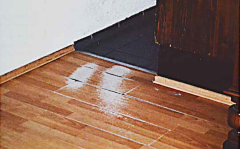
Abrasion caused by lack of barrier mats
