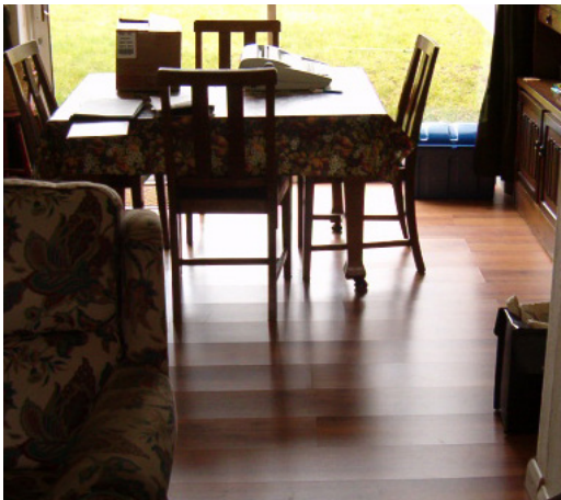
Dishing of laminate floor elements due to lack of vapour barrier (i.e. No DPM over concrete subfloor)
