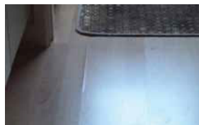
Swelling from moisture ingress
