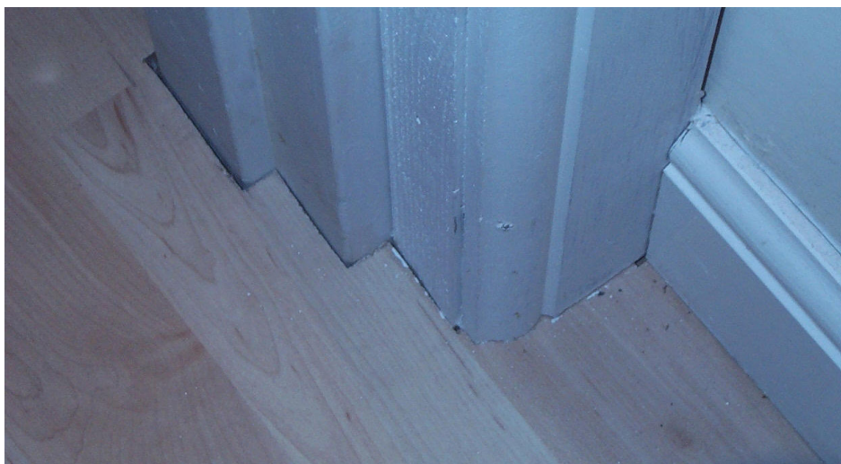
Fitting too closely to stair railing / components
