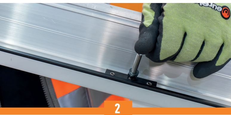
PLACE THE JACK RAFTER INTO POSITION, LOCATING THE JACK RAFTER BAR ONTO THE JACK RAFTER FIXING AND ONTO THE DOUBLE STUDS AT THE RING BEAM END. TIGHTEN ALL NUTS.
