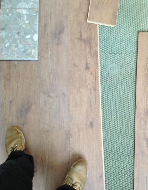
Significant difference in level of shine
