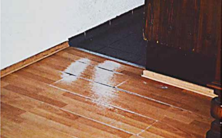
Abrasion caused by lack of barrier mats
