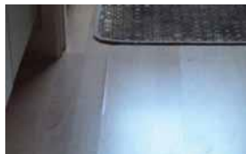
Swelling from moisture ingress
