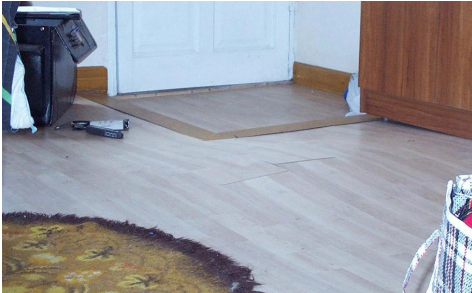
Surface temperature too high
