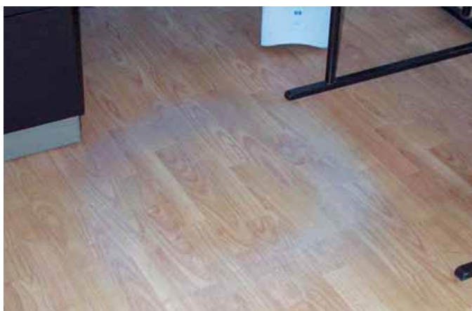
Abrasion caused by incorrect chair casters
