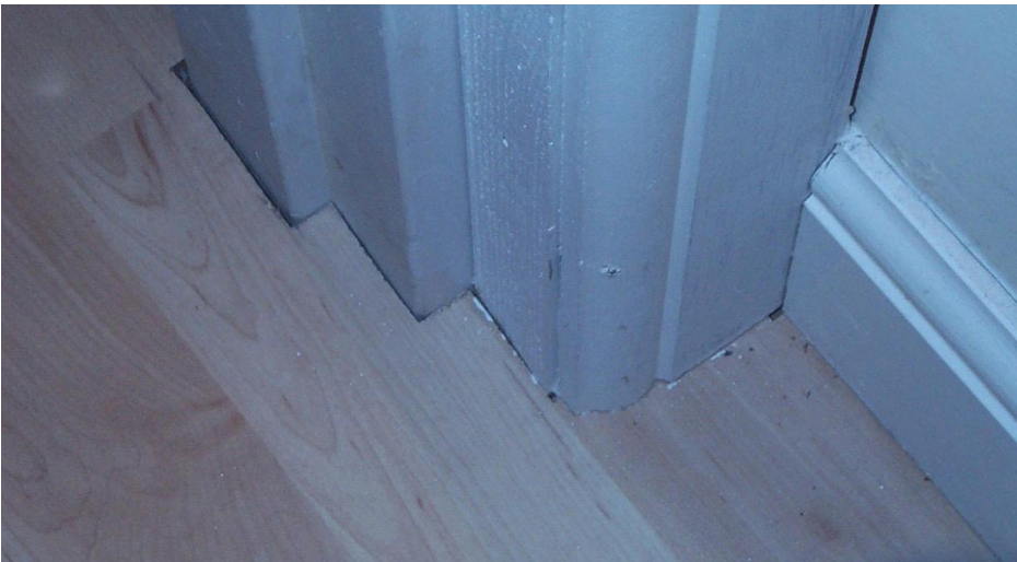
Fitting too closely to stair railing / components
