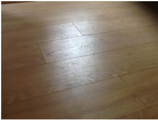
Incorrect cleaning agent/smears on the surface
