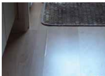
Swelling in edge area caused by moisture
