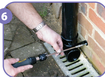
6 Fit the shoe at the bottom of the downpipe so that it directs water into the drain, if required. Secure the joint with a pipe clip.
