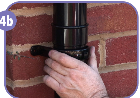
Fit the pipe clips to the downpipe and screw them into the wall.
