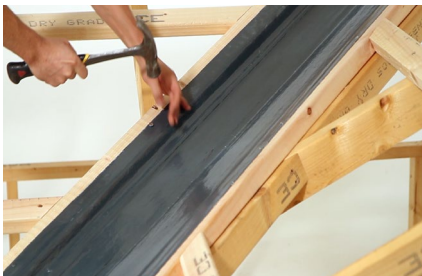
Fixing GRP valley lining Alternatively pre-formed GRP valley liners are laid between the purlin trimming battens and secured by nailing. Underlay can be dressed over the upstands.
